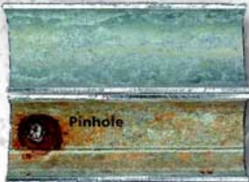
Dry Pipe Deposit
